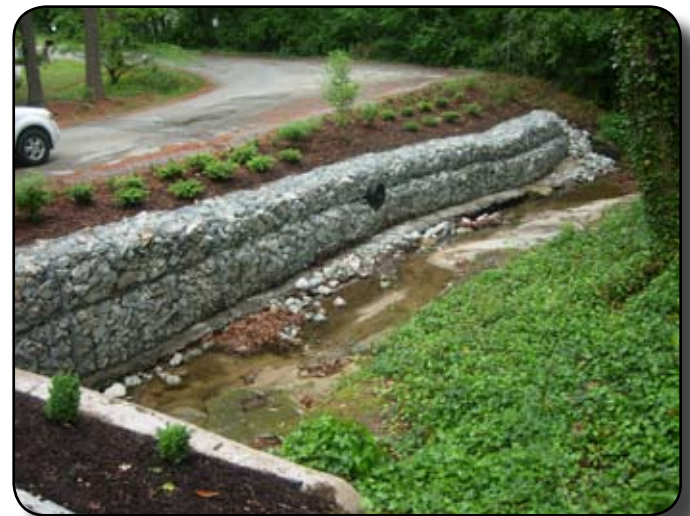
Erosion and sediment control practices on Frontier Road in the 4th District prevents the slope from washing into the ditch.
